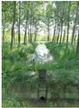
Figure II.11.6: Dehydrating ditch with latch for directing the wastewater (Photo: Zsuzsanna Uri)
