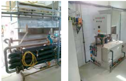
Figure II.11.9: Pipe flocculator (on the left) and polymer dosage device (on the right)
