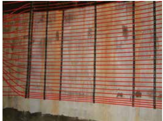
Figure III.5.4: Heating pipes inside the fermenting area
