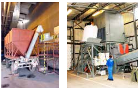
Figure II.10.27: Feeding by-products of animal origin (bone and meat meal) for combined incineration at the cement plant in bulk and big-bags (Source: Süveges, 2010)
