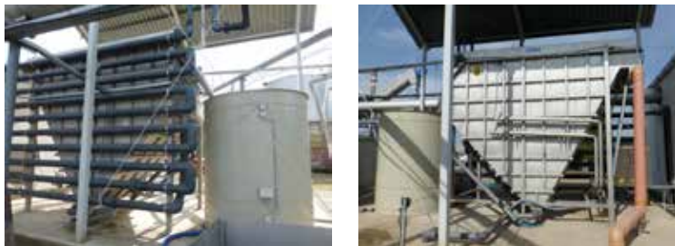
Figure II.11.3: Pipe flocculator and flotation equipment with dissolved air (DAF) (Photo: Zsuzsanna Uri)
