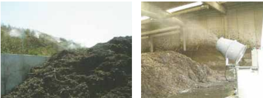
Figure III.7.11: Deodorant spraying systems
