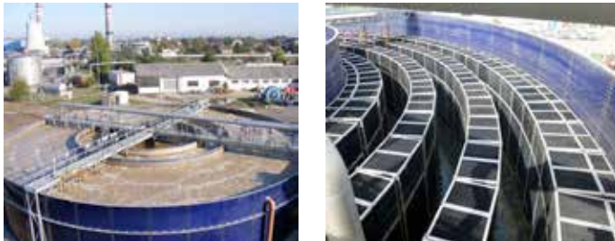
Figure II.11.2: The Flexipak ® biological wastewater treatment unit of the canning plant and the ring reactor of the Flexipak ® system (Photo: Zsuzsanna Uri)
